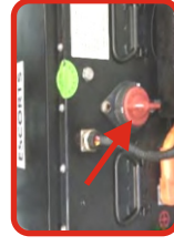
MSD switch - To Cut off the 72 Volt output from Battery
