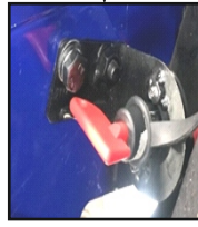
12V Battery Switch In "ON" Condition
