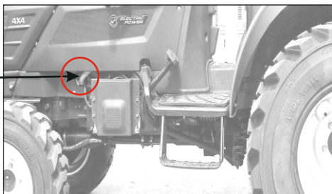
1. High Voltage Cable
