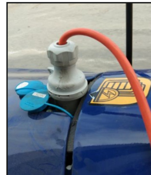
RCD Charging Cable Plugged In
